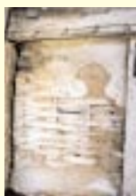
Lime-coated wattle and daub panelling is quite rare. Although poor maintenance has led to decay in this case, the damage can be repaired
