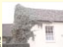
Climbing plants trap moisture against the building and can lift or crack roof coverings
