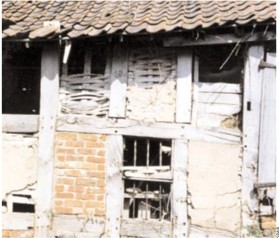
A decayed timber framed wall with infill panels of original wattle and daub and later brick
