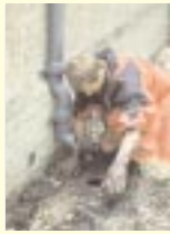
Rainwater gullies should be regularly cleared of blockages such as dead leaves
