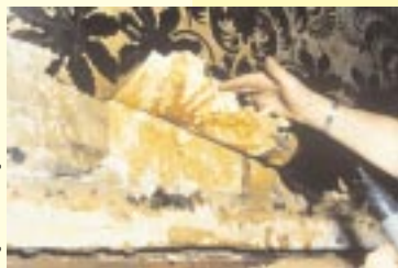
Historic decoration is sometimes revealed during the course of repair work. Here, a conservator salvages a fragment of historic wallpaper
