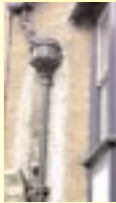
A blocked downpipe has leaked, causing damage and staining to the brickwork and encouraging the growth of vegetation
