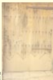
Careful piecing-in of new timber to repair the base of an early oak door
